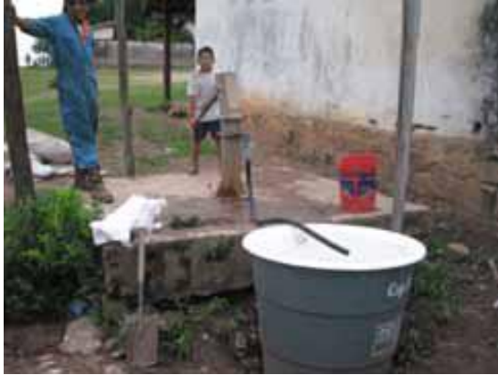
Pump for groundwater and source water tank
